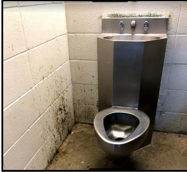
Figure 2: Photo of Mold in Camp J Shortly After Camp Closure.
